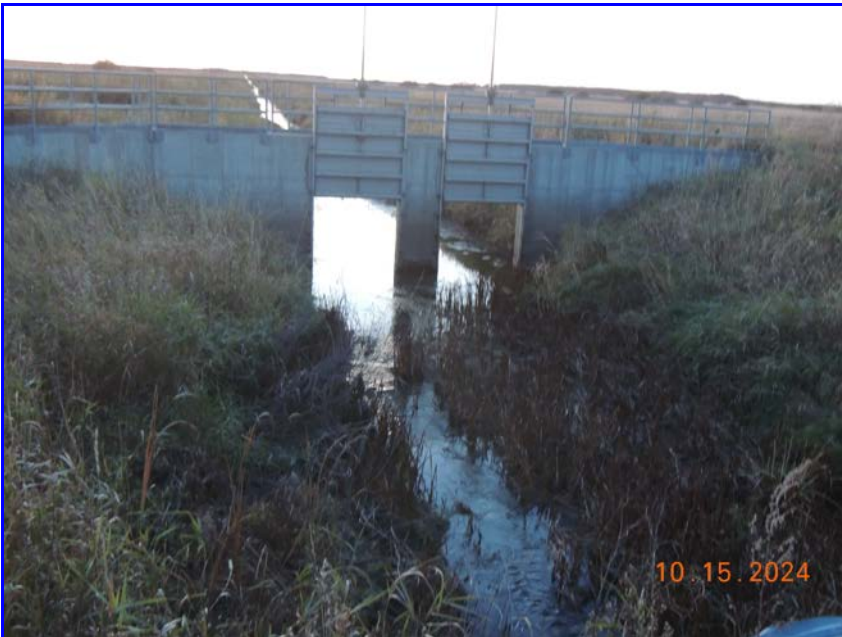
Photo 12 - Closer view of the outlet gates and stilling basin at the northeast inlet structure.
