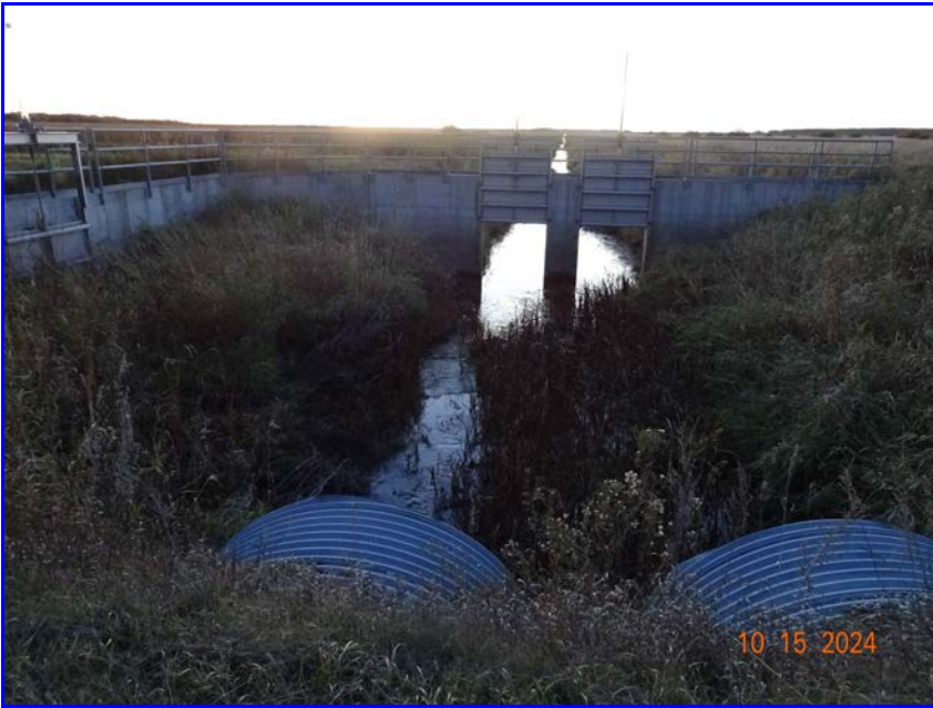
Photo 11 - Northeast inlet structure: Looking downstream at the stilling basin and outlet control structure to the west. The two conduits shown are the downstream end of the impoundment inlet.
